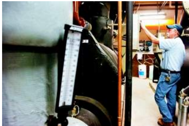
BYRON ELLIS WORKS on an HVAC system at the University of Southern Mississippi. The university plans to shut down the system over spring break to conserve energy. HVAC is a system for heating and cooling. (ERIN PARKER | Hattiesburg American)
